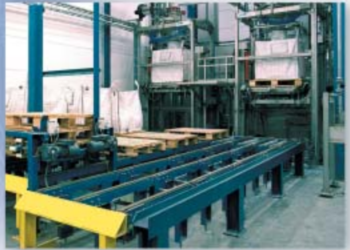
■ Big-Bag filling system for handling resin flakes
